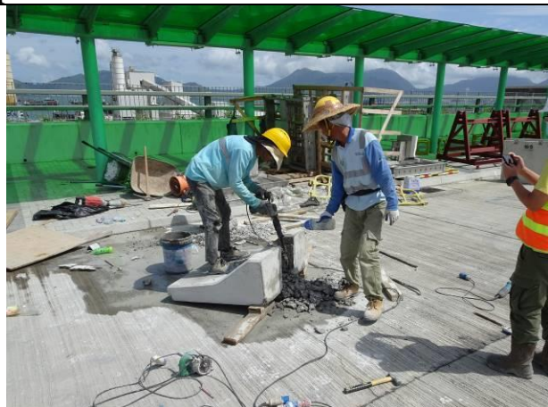
Photo 9 During the joint site inspection on 16 June 2020 water spraying had been provided for breaking works to reduce dust impact.
