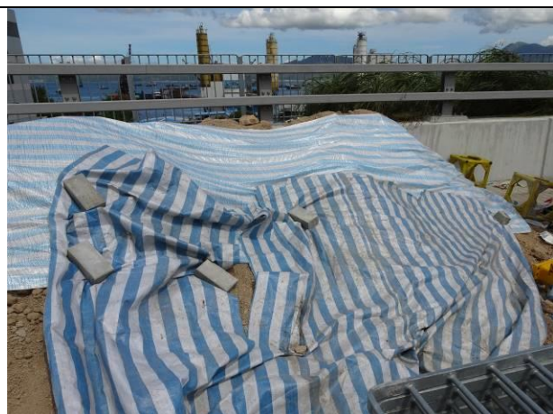
Photo 8 During the joint site inspection on 9 June 2020 stockpile of loose material had been covered with tarpaulin to reduce dust impact.
