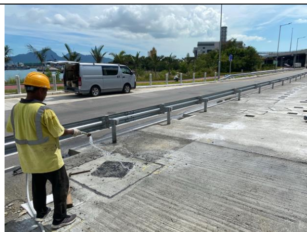
Photo 8 During the joint site inspection on 11 August 2020 water spraying had been provided for the exposed area to reduce dust impact.
