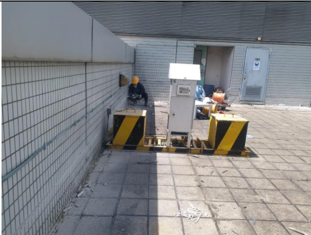
Photo 15 Renovation works was undertaken at the root top near the monitoring station of ASR6 (Taken by ET of HY/2012/08)
