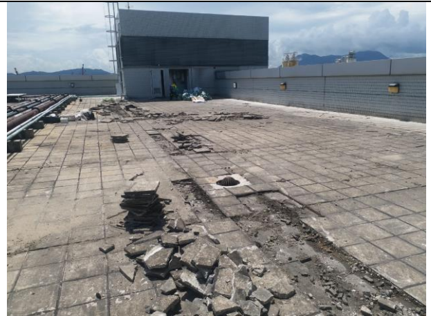
Photo 16 Renovation works was undertaken at the root top near the monitoring station of ASR6 (Taken by ET of HY/2012/08)
