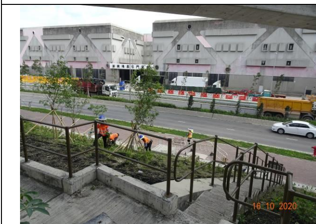
Photo 9 During the joint site inspection on 16 October 2020 landscape works was undertaken at Lung Mun Road and no dust emitted from the site activities was observed.
