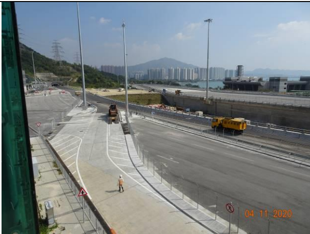
Photo 9 During the joint site inspection on 4 November 2020, no dusty activities were observed from the site near the monitoring station.
