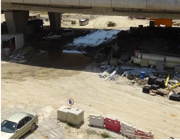
Photo 7 All vehicles using the haul road had enhanced to control the speed below 8km/hr to reduce dust emission.
