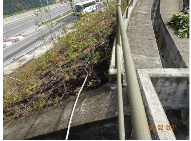
Watering system at Slope TP_C
