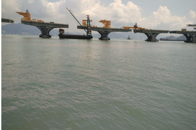
Photo 10 - Mid-Flood at IS8 on 11 September 2017
