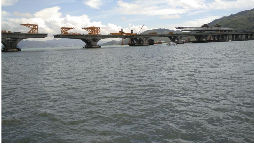
Photo 1 - Mid-Flood at IS8 on 25 September 2017
