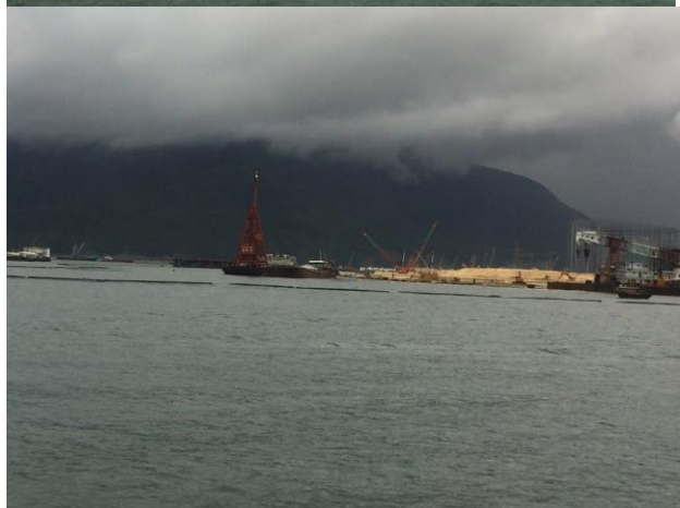
5.1.8.17 Photo record taken on 25 June 2015 shows that no silt plume around Portion E1 of HKBCF reclamation works were observed during the site inspection conducted on 25 June 2015.
