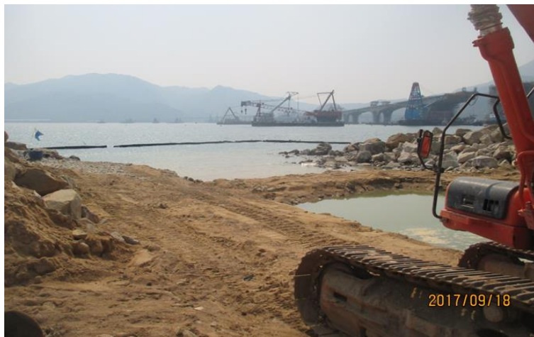
Photo record shows silt curtain condition and active works area at outfall area on 18 September 2017.
