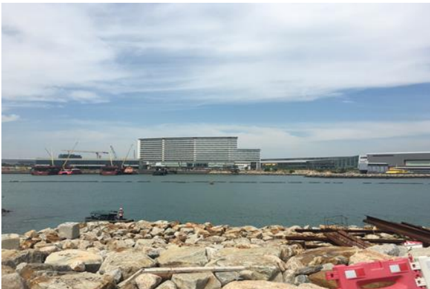
Photo record shows silt curtain condition at active works area of seawall construction on 14 September 2017.
