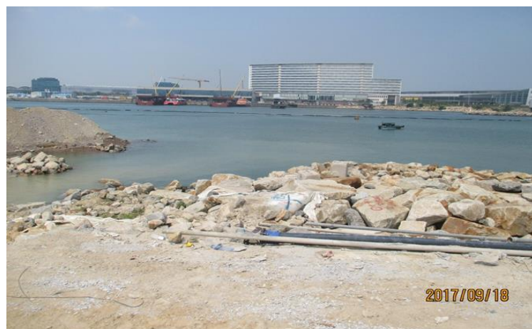
Photo record shows silt curtain condition and active works area at seawall construction area on 18 September 2017.
