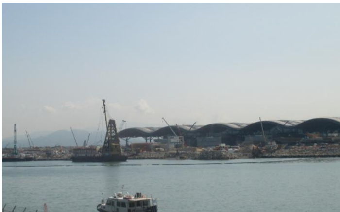
Photo record shows silt curtain condition and active seawall construction area on 28 September 2017.
