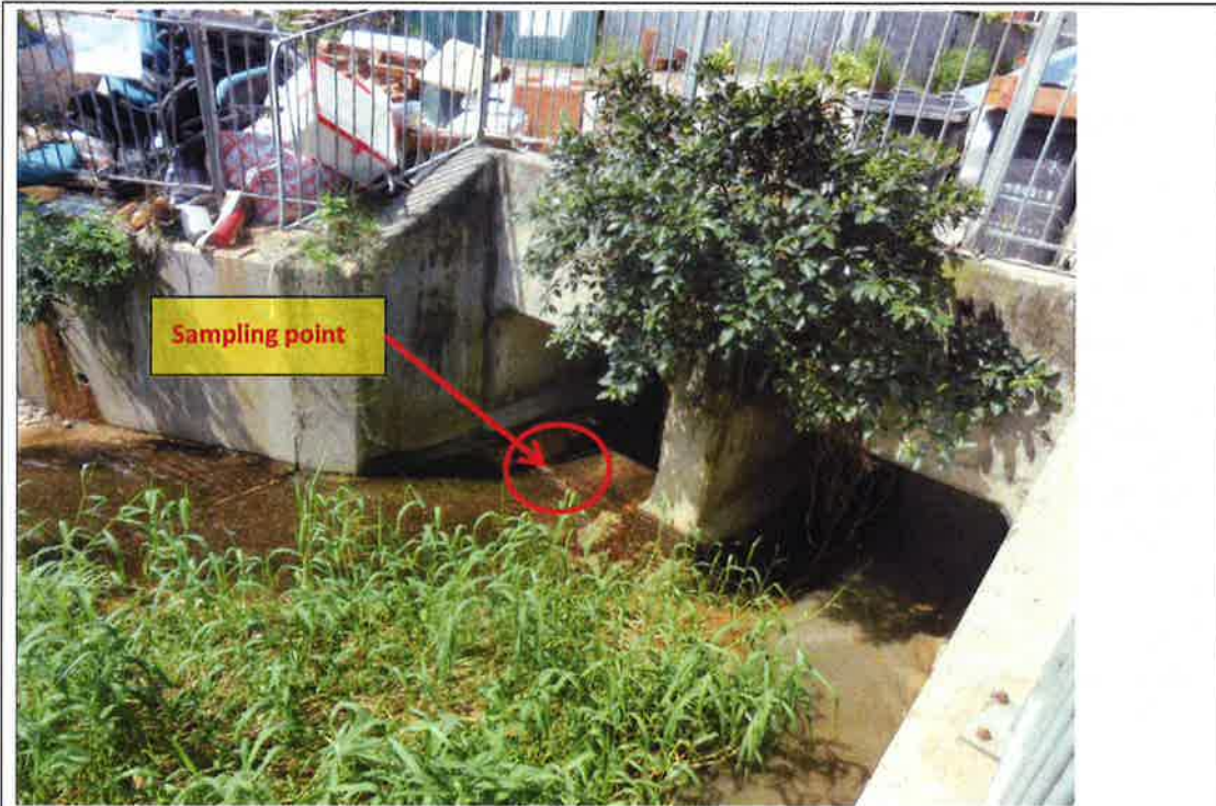
Photo 1 Location WM2B (under the bridge) The water depth of WM2B is approximately 0.01-0.02m
