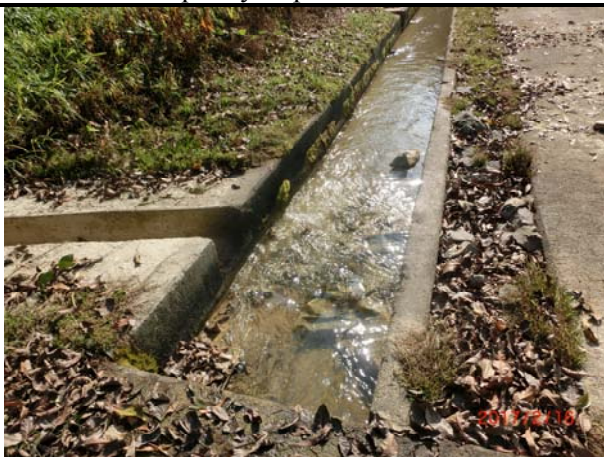
Photo 5 During site inspection on 16 February 2017 at WM3x of Ng Tung River, it was observed that water flowing at WM3x was clear.
