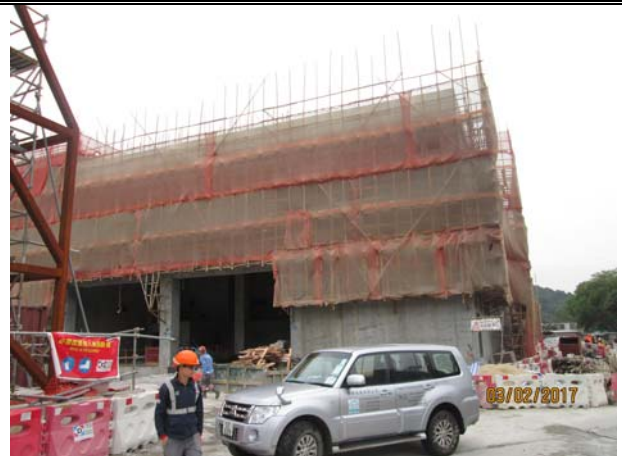
Photo 4 Superstructure works for Admin Building was carried out and wastewater generated from the site was limited. The site area was mostly hard paved and no adverse water quality impact was identified.
