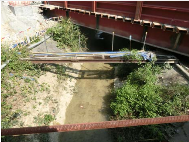
Photo 3 On 13 February 2017, inspection was carried out at downstream of South Portal works area of Contract 6, it was observed that the water flowing from the construction site was visually clear and no adverse water quality impact was observed.
