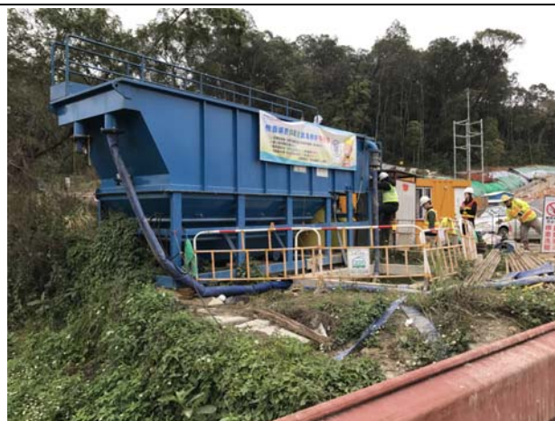
Photo 6 A wastewater treatment facility with AquaSed SH-20 was implemented.
