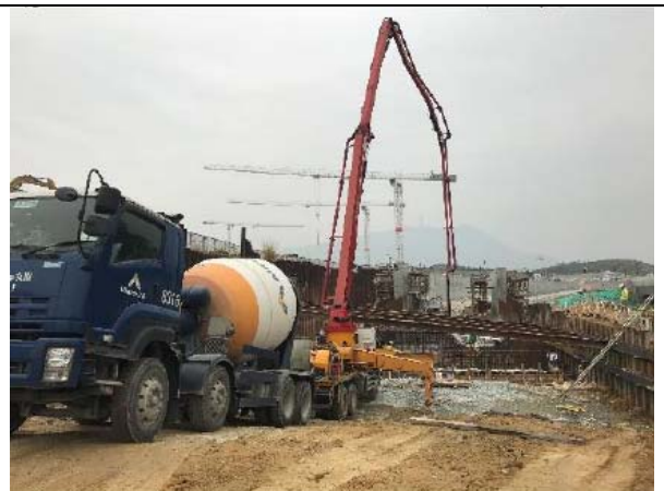
Photo 5 During site inspection in February 2017, it was observed that the main construction activity was construction of depressed road near Bridge Y and no adverse water quality impact was recorded.
