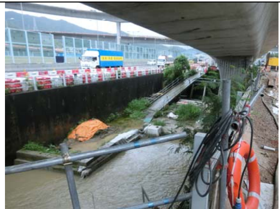
Photo 10 During weekly site inspection by ET on 6 July 2017 at the works area adjacent to river channel, no adverse water quality impact was observed with the mitigation measures implemented by the Contractor. However, turbid water was observed in the existing river channel under the influence of rain.
