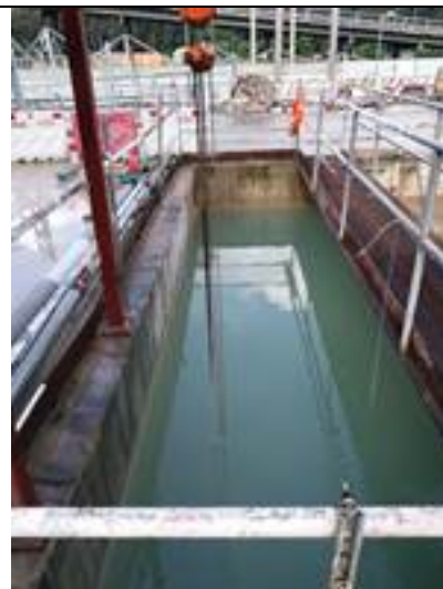
Photo 12 DHK daily record on 8 July 2017 shown the discharge quality in South Portal was in acceptable condition.
