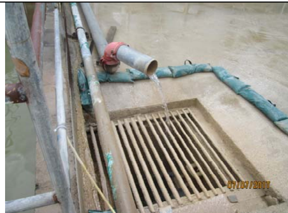
Photo 10 During weekly site inspection at South Portal by ET on 7 July 2017, it was observed the wastewater treatment facility implemented on site was function properly and the discharge water from the site was clear.
