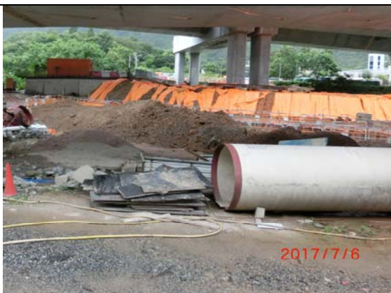
Photo 11 During weekly site inspection by ET on 6 July 2017, it was observed that the slope adjacent to river channel was covered with tarpaulin sheet to minimize muddy runoff.
