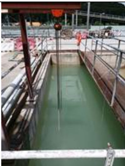
Photo 11 DHK daily record on 6 July 2017 shown the discharge quality in South Portal was in acceptable condition.
