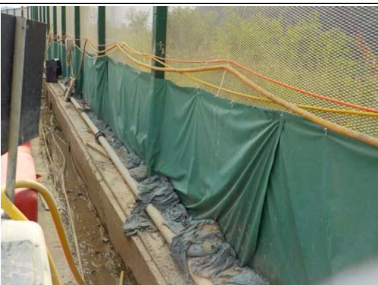
Photo 5 During rainy day, the surface runoff would be collected by the temporary drainage and all the wastewater generated from the site including runoff would be passing through the perimeter channel and diverted to the wastewater treatment plant for treatment before discharge.
