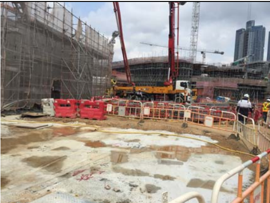
Photo 3 During site inspection on 4 October 2017, it was observed that wastewater generated from the active construction activities was limited.
