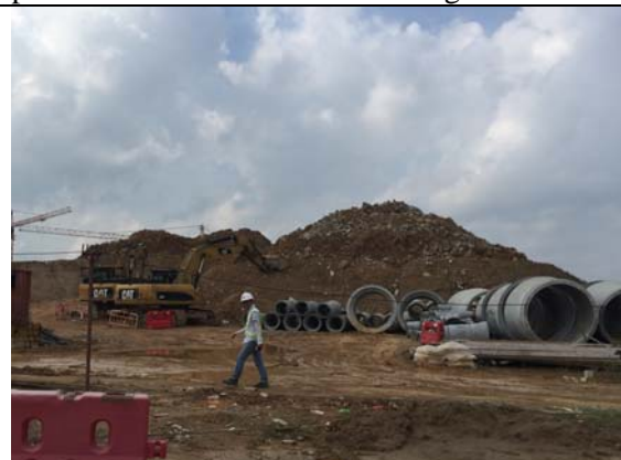
Photo 6 Exportation of the stockpile was in progress in which the stockpile was compacted after excavation and the runoff generation from the stockpile would be collected by the temporary site drainage as well.
