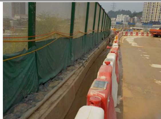
Photo 4 During rainy day, the surface runoff would be collected by the temporary drainage and all the wastewater generated from the site including runoff would be passing through the perimeter channel and diverted to the wastewater treatment plant for treatment before discharge.
