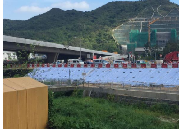
Photo 16 The exposed slope next to the river channel was covered with impervious sheet to minimize generation of muddy runoff flowing into the channel.
