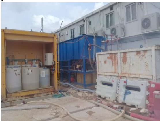
Photo 11 The wastewater treatment facilities were implemented as per the temporary site drainage plan.
