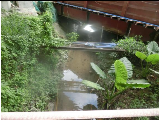
Photo 9 Upon detection of the exceedance on 4 July 2018, inspection was carried out at the river channel crossing of works area of Contract 6 and it was observed that water flowing from site area of Contract 6 was clear.
