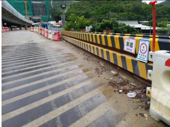
Photo 15 The site area adjacent to the stream was completely sealed to minimize the risk of site runoff flowing into the exiting stream.
