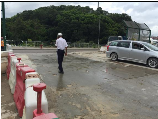
Photo 9 During site inspection at the site exit on 18 July 2018, no site runoff flowing from the site to public area was observed.
