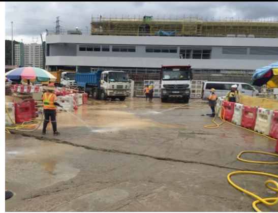
Photo 8 Wheel washing facility was implemented at the site exit (Gate 3), a ditch was constructed to collect the wastewater generated by wheel washing for recycling purpose.
