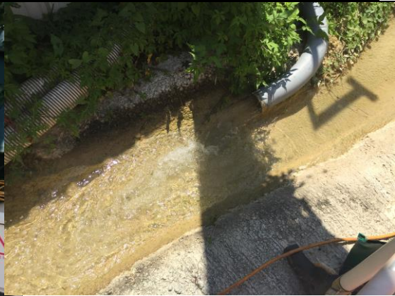
Photo 14 Wastewater treatment facilities at South Portal were function properly and the effluent was clear.
