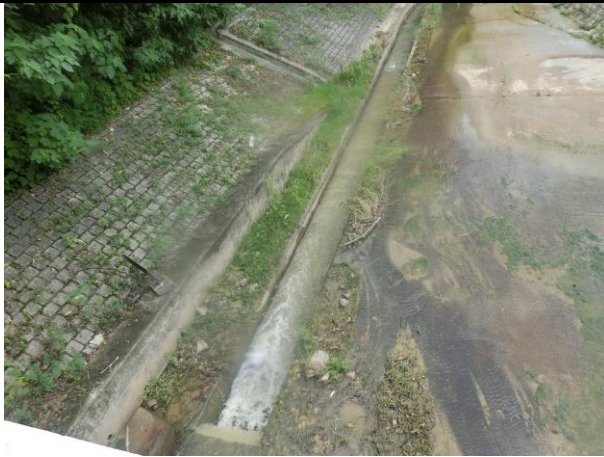
Photo 7 During water sampling on 9 July 2018, the water quality observed at WM3x was turbid.
