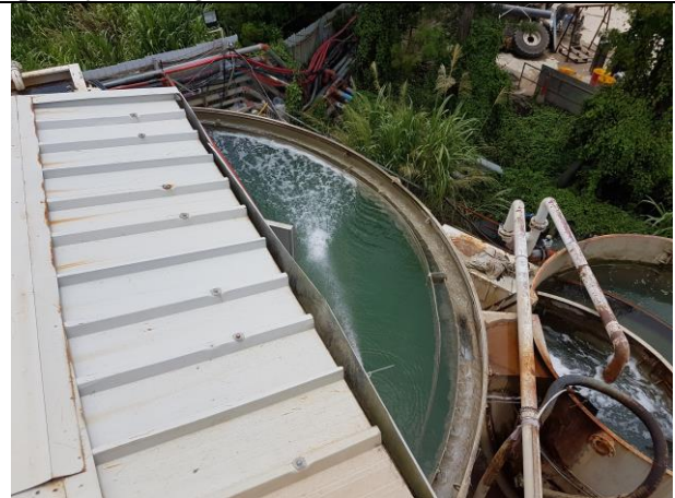
Photo 10 During site inspection on 6 July 2018, it was observed wastewater treatment facilities were in place properly.
