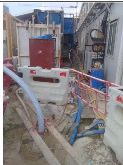
Photo 12 During rainy day, the surface runoff from the site will be collected by the temporary drainage which built according to the temporary site drainage plan. All wastewater generated from the site will pass through the perimeter channel and divert to the wastewater treatment facilities for treatment prior to discharge.
