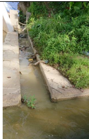
Photo 12 As reported by the CCKJV, inflow of turbid water was occasionally observed from the open channel which receiving the stormwater from the Sha Tau Kok Road.
