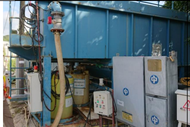
Photo 13 Joint site inspection was conducted on 5 July 2018. It was observed that wastewater treatment facilities at South Portal were function properly.
