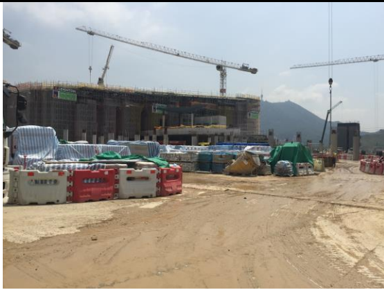
Photo 7 During site inspection on 11 July 2018, it was observed that wastewater generated from the active construction activities was limited.
