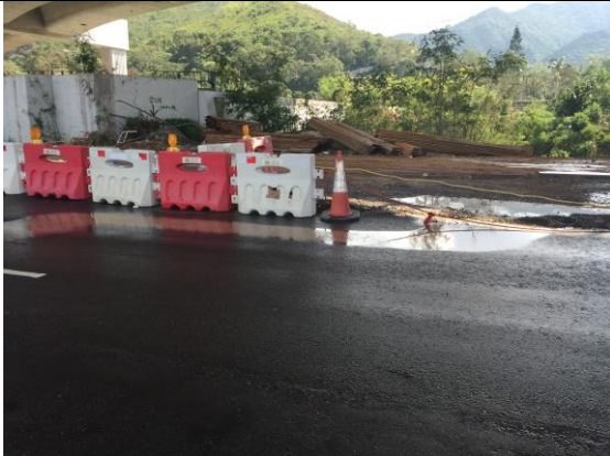
Photo 3 Based on ET's site inspection record in September 2018, overflow of wastewater from wheel washing to public road was observed at work area of site exit SA2. The Contractor was advised to clean the muddy water and provide proper mitigation to avoid muddy water flow out of site.
