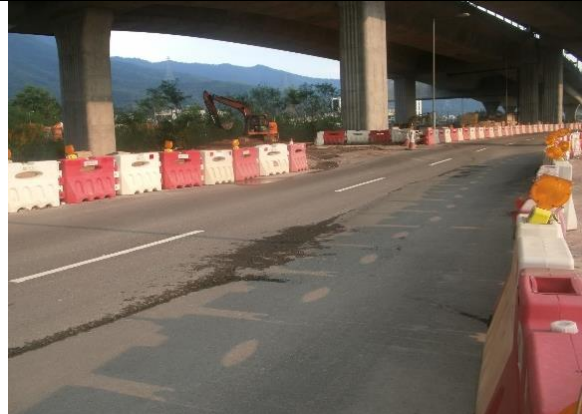
Photo 4 The muddy water at public road was cleaned and Chun Wo was reminded to improve the condition of site exit.
