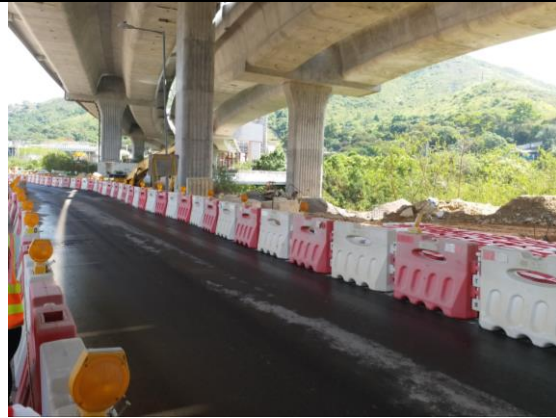
Photo 2 Road cleaning by water tanker as dust suppressive measure was observed on Tai Wo Service Road East.
