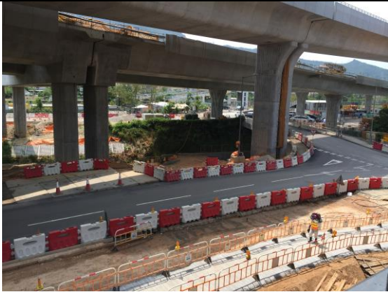
Photo 1 During site inspection on 3 May 2018, no adverse impact was observed on Tai Wo Service Road East and there was no site exit along the road under the Project.
