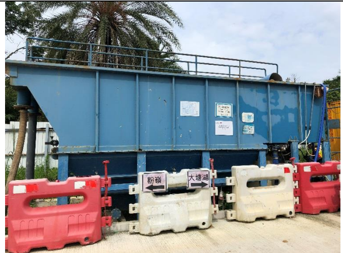
Wastewater treatment facility was implemented.
