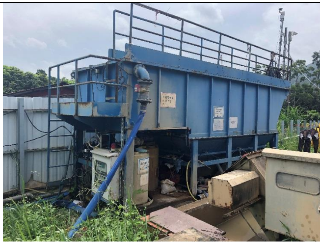
Wastewater treatment facility was implemented.
