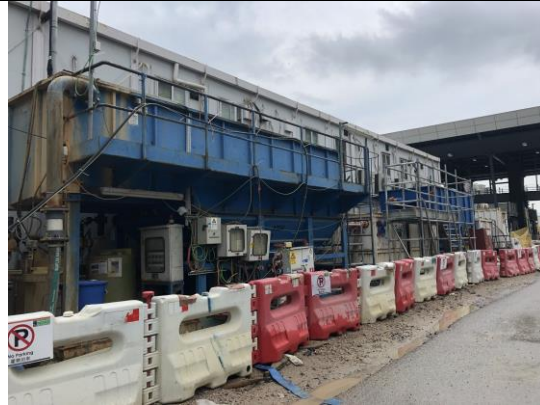
Wastewater treatment facility was implemented.
