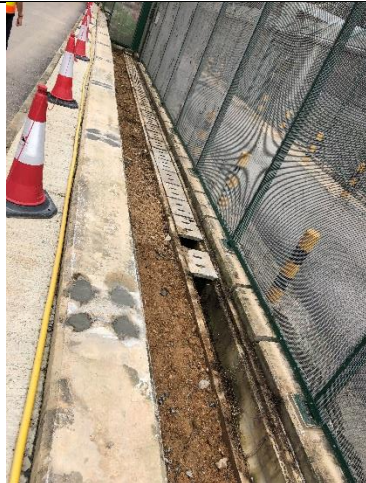
Perimeter channel to collect site runoff.
