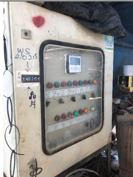
Wastewater treatment facility was properly implemented.
