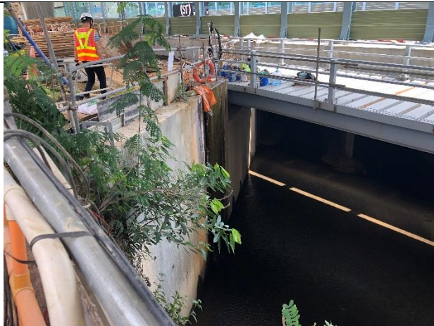
The discharge from wastewater treatment facility was clear.
