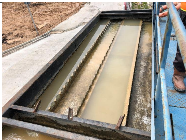
No milky water was observed and the wetsep was maintained in good condition.
