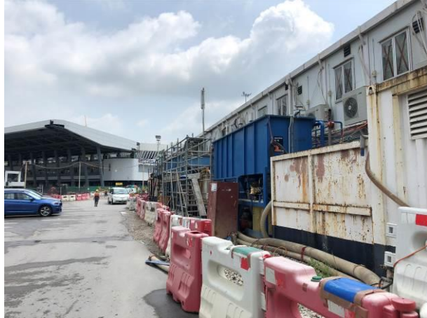
Wastewater treatment facility was implemented within site area.
