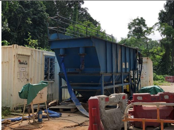
Wastewater treatment facility was implemented.
