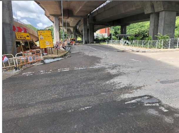
No wastewater flowing from the site to public road was observed.
