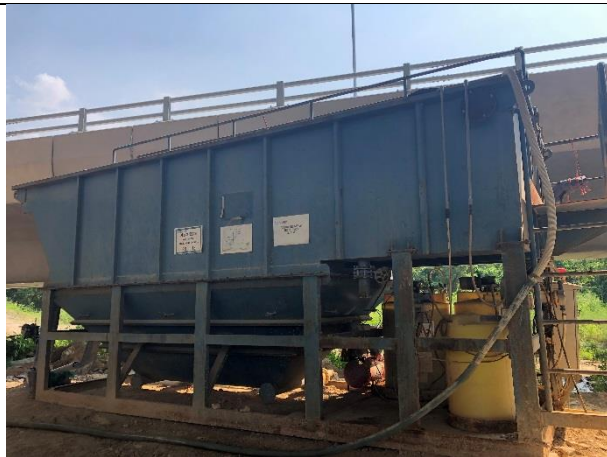
Wastewater treatment facility was implemented.
