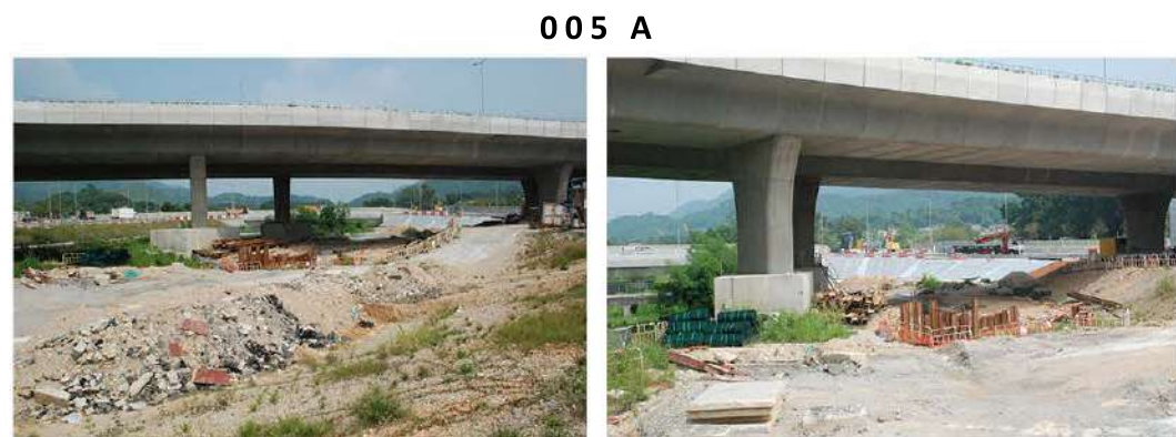
005 A Buffer Trees Planting with Amenity Shrubs Planting (OM3 & 4) Tree Planting on Landscape Slope (OM3 & 7)
