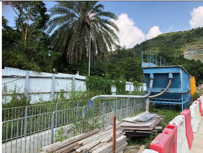
Wastewater treatment facility was implemented.
