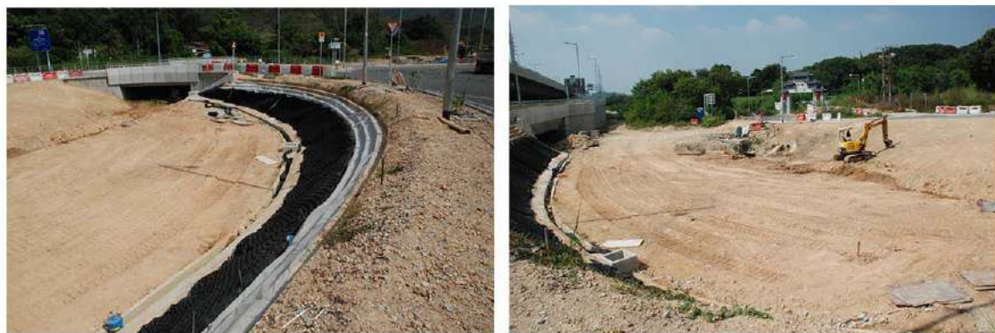
Buffer Trees Planting with Amenity Shrubs Planting (OM3 & 4) Amenity Roadside Trees Planting (OM3 & OM10)
