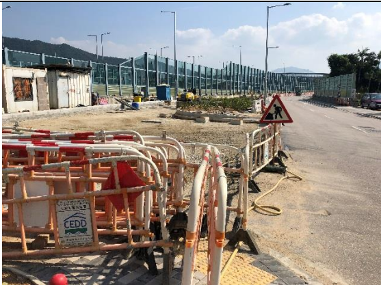
The exit was no longer used as a site exit.
