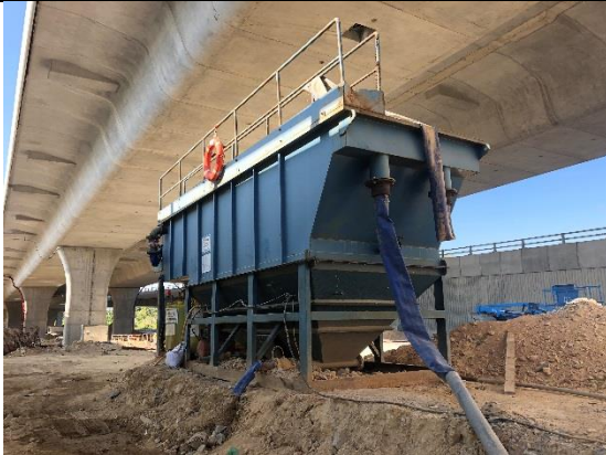
Wastewater treatment facility was implemented
