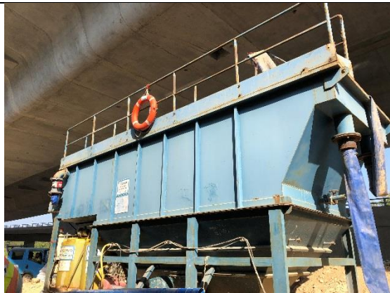
Wastewater treatment facility was implemented
