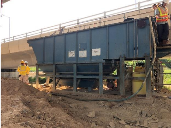
Wastewater treatment facility was implemented
