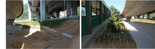
Tree Planting on Landscape Slope (OM3 & OM7) Amenity Roadside Trees Planting (OM3 & OM10) Shrubs and/ or Groundcover Planting (OM10)
