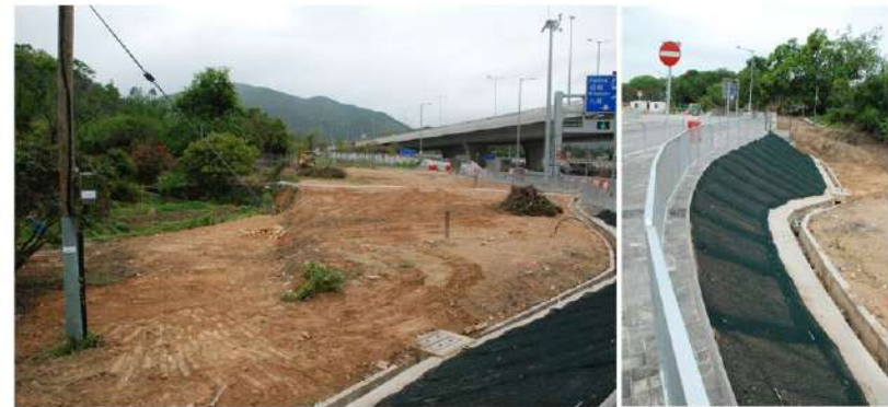
Buffer Trees Planting with Amenity Shrubs Planting (OM3 & 4) Amenity Roadside Trees Planting (OM3 & 10) Hydroseeding on Slope (OM7)
