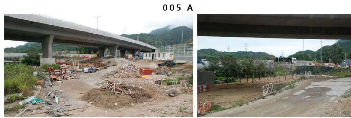
005 A Buffer Trees Planting with Amenity Shrubs Planting (OM3 & 4) Tree Planting on Landscape Slope (OM3 & 7)
