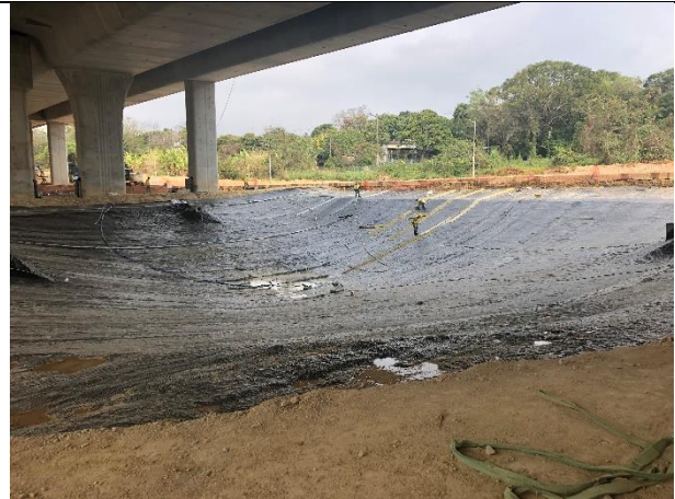
Photo 2 The exposed surface was covered with waterproof membrane at proposed pond at WCA.
