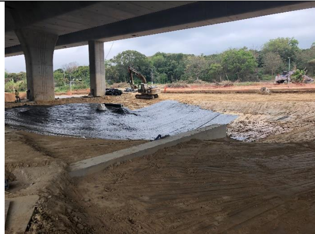
Photo 2 The exposed surface was covered with waterproof membrane at proposed pond at WCA.
