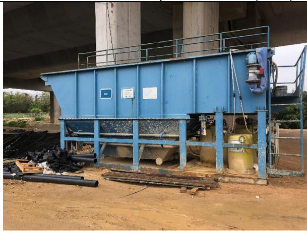
Photo 3 Wastewater treatment facility was implemented at WCA.
