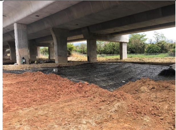
Photo 2 The exposed surface was covered with waterproof membrane at proposed pond at WCA.
