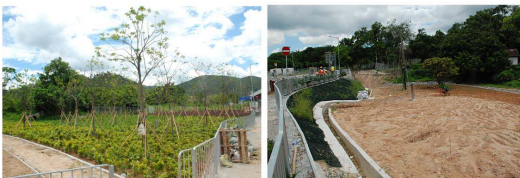
Buffer Trees Planting with Amenity Shrubs Planting (OM3 & 4) Amenity Roadside Trees Planting (OM3 & 10) Hydroseeding on Slope (OM7)
