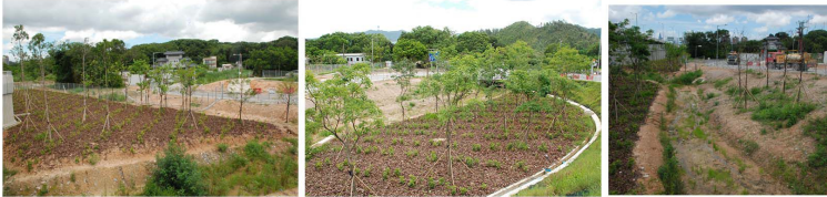
Buffer Trees Planting with Amenity Shrubs Planting (OM3 & 4) Amenity Roadside Trees Planting (OM3 & OM10)
