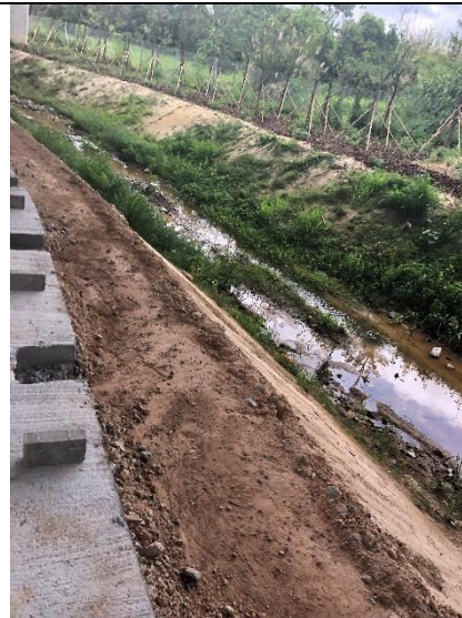
Photo 2 The water quality of the stream adjacent to the site was clear.
