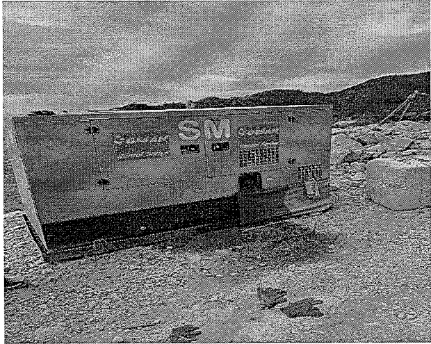
Photo 211215_001 (Near the generator)
