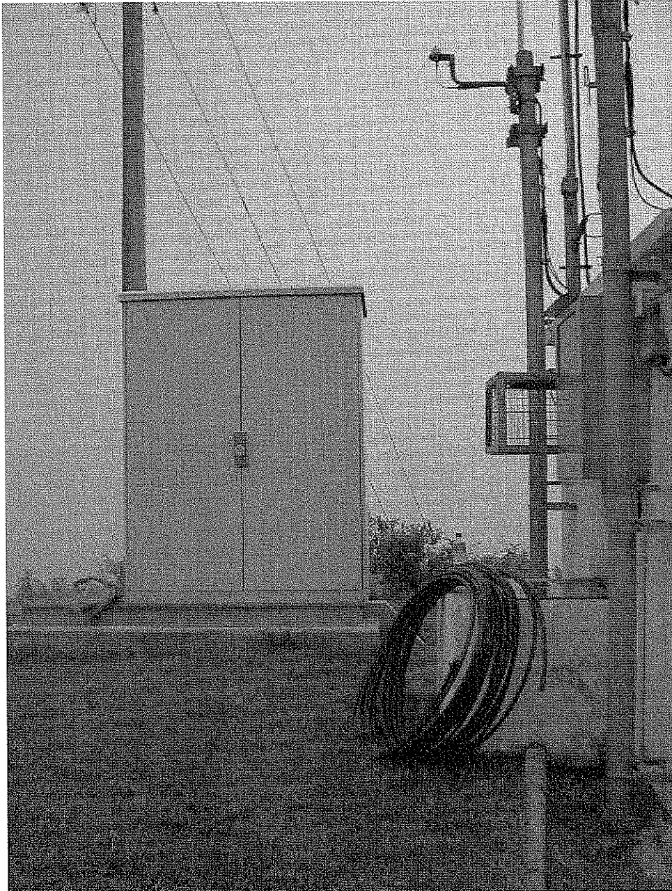
Picture 3: General View of the HKPF Radio Equipment
