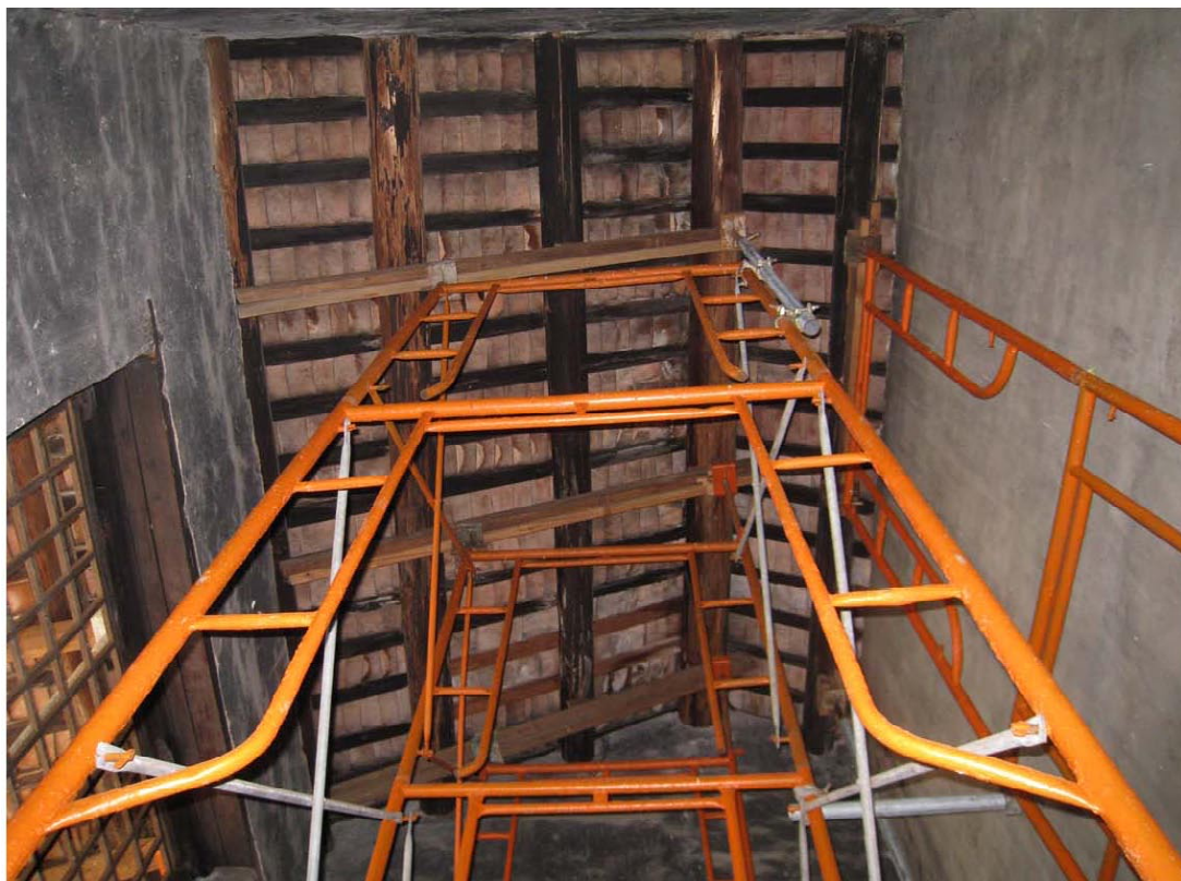
Plate 2 Purlins in the Ancestral Hall have been seriously damaged.
