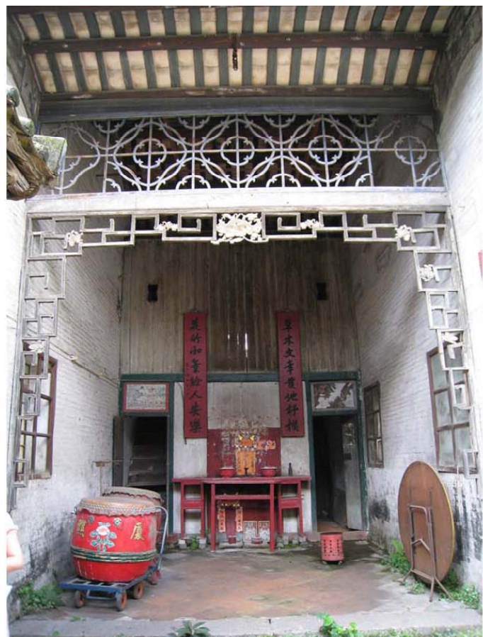
Plates 5 & 6 Repair to floor tiles throughout the Tang Ancestral Hall and Guest House is required.
