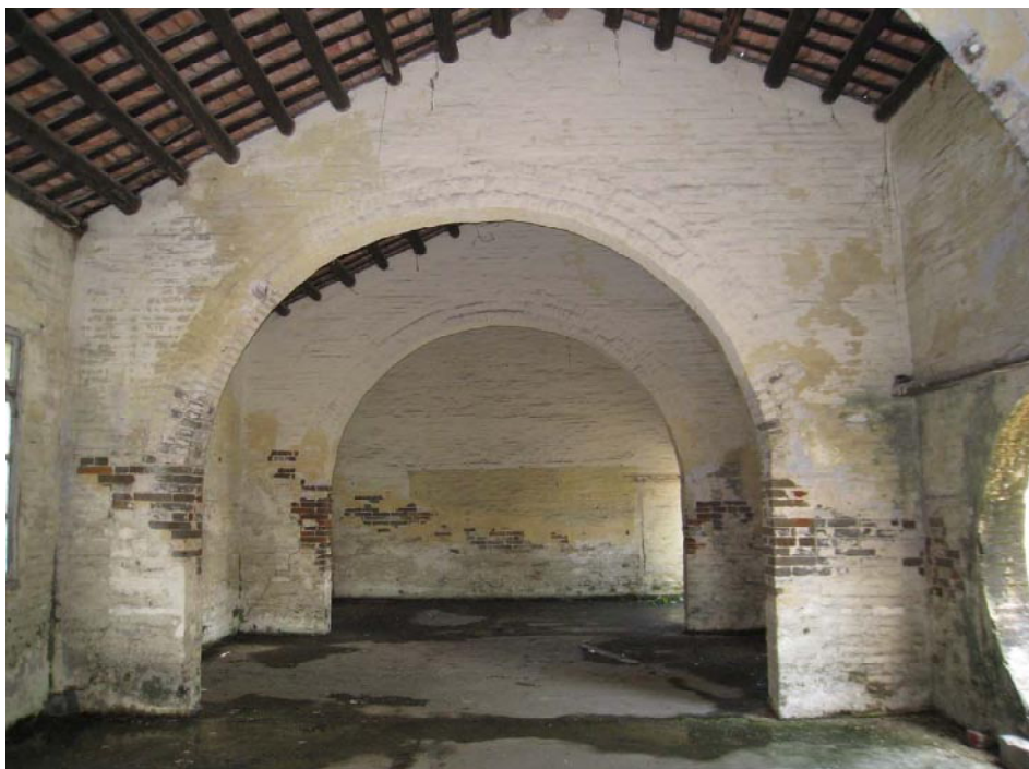
Plate 10 Removal of the existing paint work to walls throughout the Yau Kung School is required.
