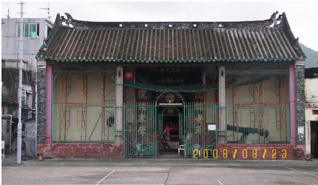
Plate 1 The front elevation of the Tang Ancestral Hall. Temporary propping has been erected by AMO. Modern paint on the walls and columns will be removed in the restoration.
