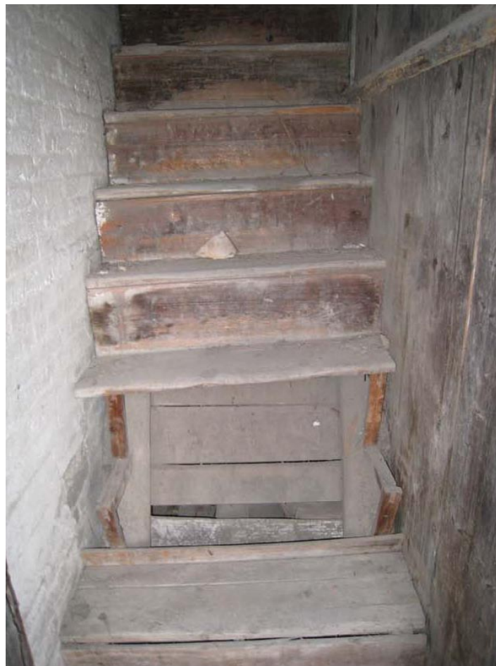
Plate 8 The timber staircase and cockloft floors at the Guest House are dilapidated.
