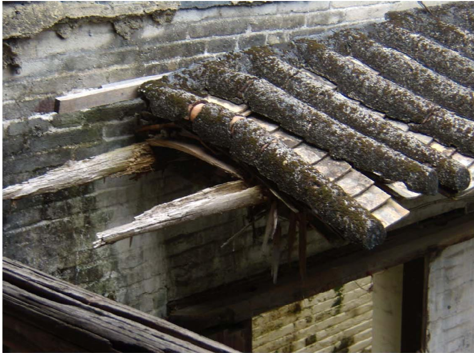
Plate 7 Defective / loosen roof tiles and battens at the Guest House
