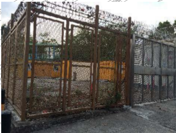
PHOTO 2: EXISTING ELECTRIC SUBSTATION (DATE TAKEN: 1 APRIL 2015)
