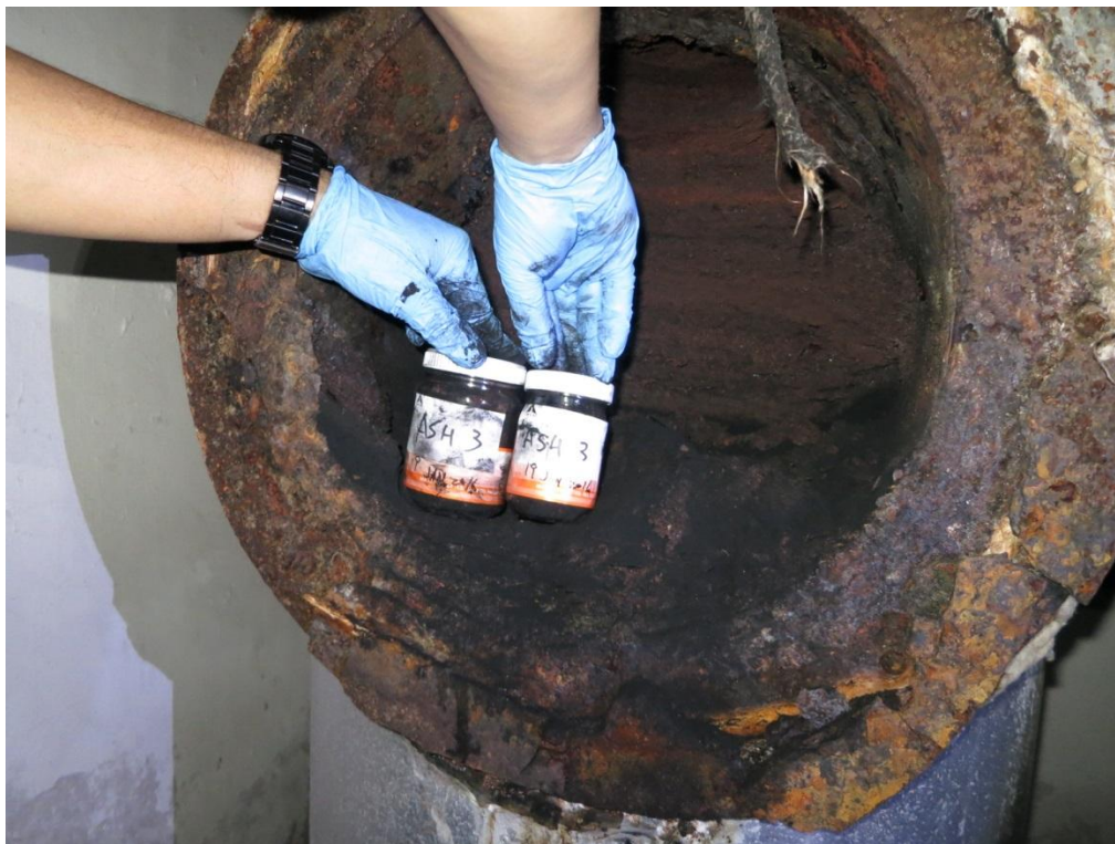
Plate 2 Residual ash sample at the bottom of chimney
