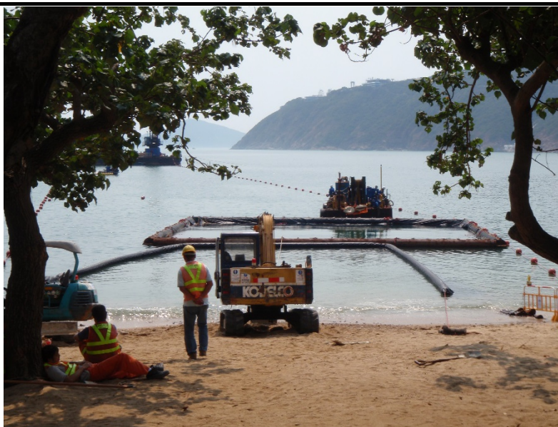
Figure 4.1 Example of silt curtains for burial works at water line and off-shore diver working area for land base work on the beach and marine based activities near shore respectively
