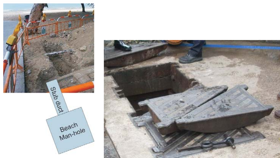
Figure 2.7 Typical Onshore Works Conditions - Trench to duct/ conduit and Opened Beach Manhole
