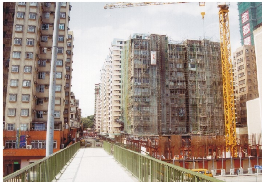
3. Typical View of High-Rise Residential 3 (HR 3) showing the older development of Jubilant Place
