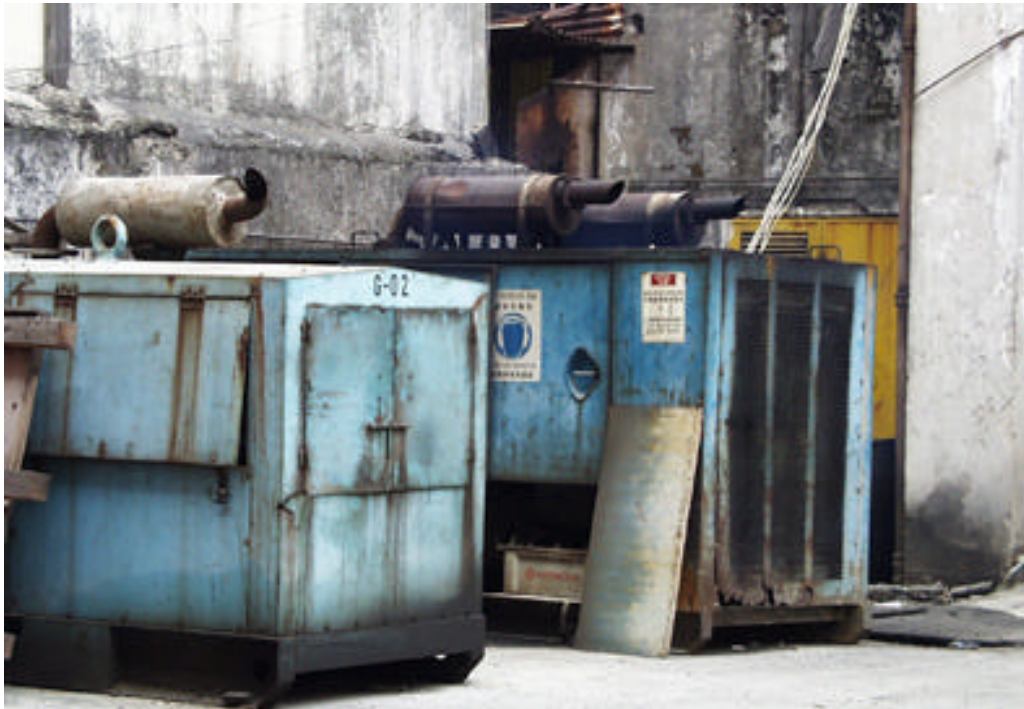
Photo 15 YTML 12 : Two operating generators on site (24 Dec 98)
