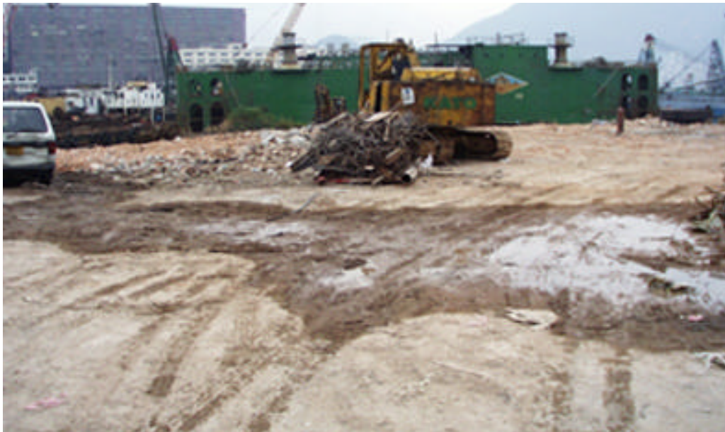
Photo 86 YTML 41-43 : Vacated site of the former ship repair workshop, former structure demolished (24 Dec 98)
