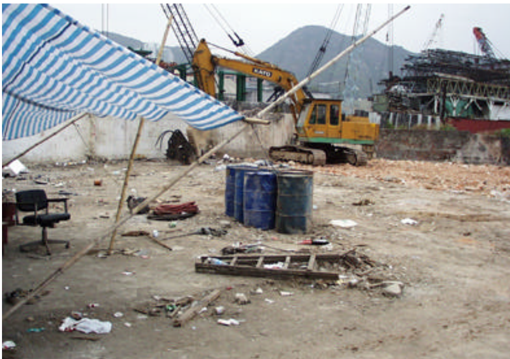
Photo 84 YTML 41-43 : Vacated jetty of the former ship repair workshop, former structure demolished (24 Dec 98)
