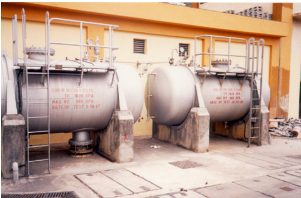
Photo 99 Two Surge Vessels Outside the Pumping Station (17 Mar 99)
