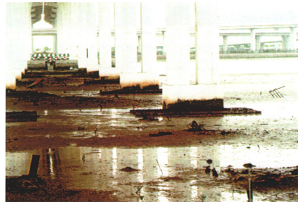
(d) View of poor quality mudflat restoration beneath Lotus Bridge, showing construction debris (wheel barrow, trolley, pipe), uneven mud surface, and pile caps above mud surface.
