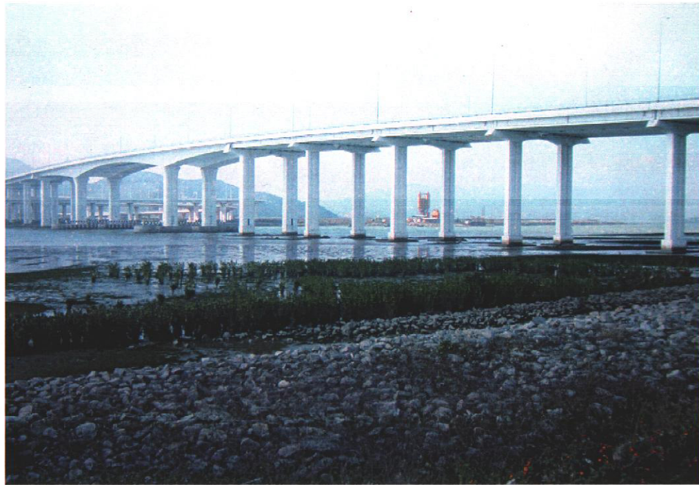
(a) Lotus Bridge viewed from southeast, showing arched sections over navigation channel, 35m pier spacing, mangrove plantation on mudflat (foreground), and inundated mudflat (behind mangrove).
