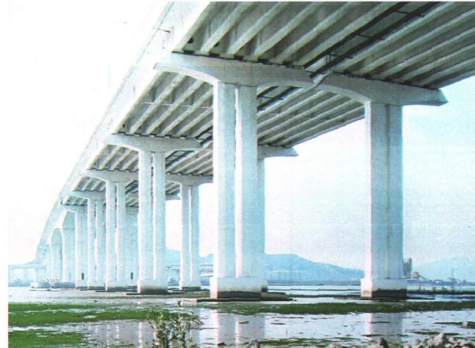
(b) Lotus Bridge seen from below, showing pairs of piers, pile caps above mud surface, and slope-covered mudflat.
