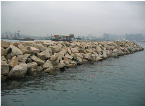
Breakwaters made of rock armour at New Yau Ma Tei Typhoon Shelter.
