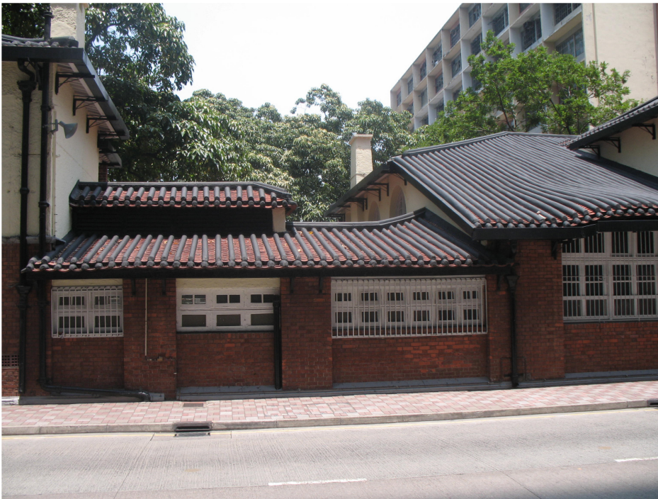
Close up of central rear section of the former Yacht Club House (前香港皇家遊艇會會所) at Electric Road (HATS-01)
