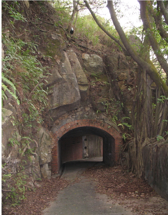
View tunnel with brick arch on the gun road leading to the old West Battery 設置在運送槍炮往前西炮台的通道之磚砌拱門隧道
