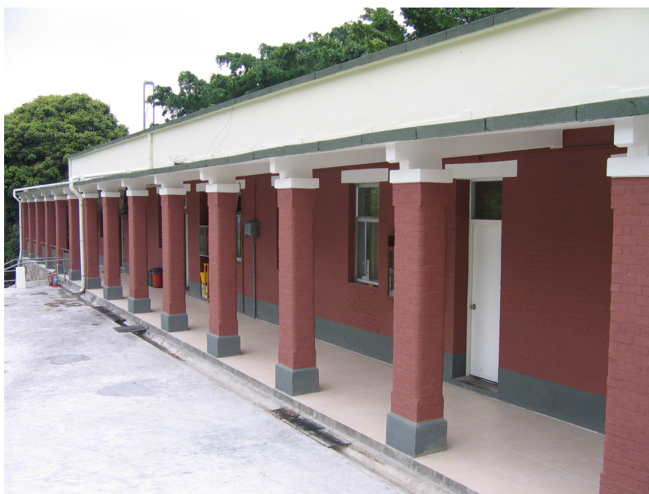
View of the façade of Block 36 (Old West Battery) 第三十六座(舊西炮台)
