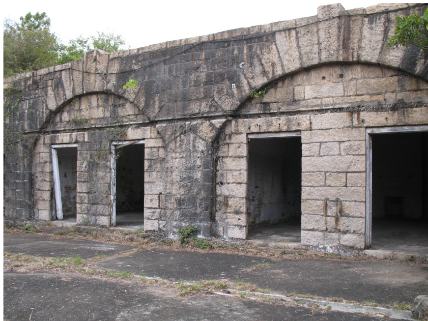
View of the ruins of magazines associated with the former West Battery 前西炮台軍火庫遺址
