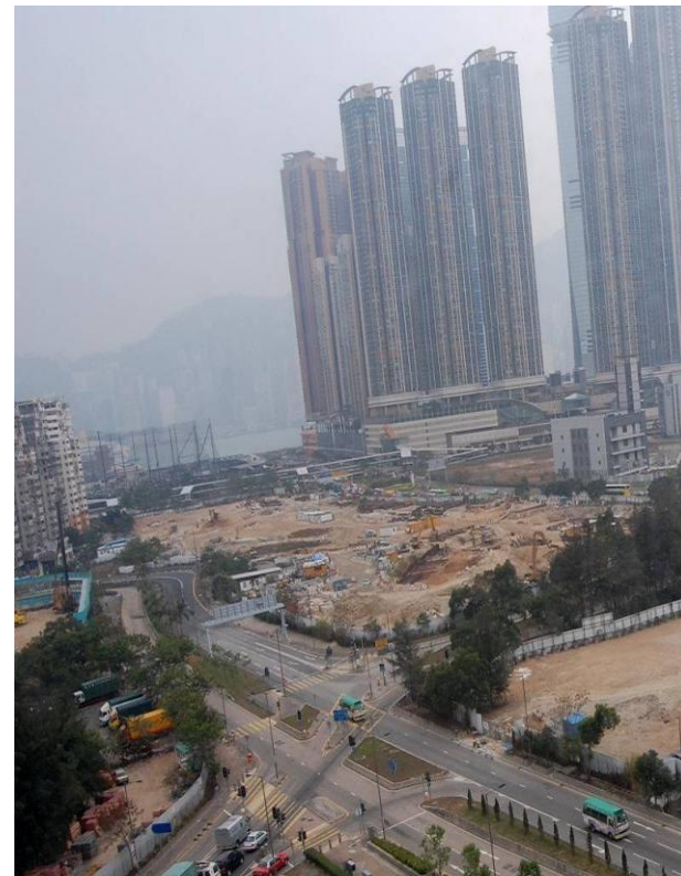
Mong Kok West Ventilation Building (MKV)
