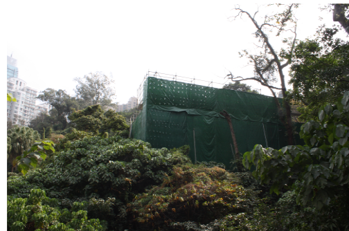
Plate 8c View of the area under renovation at the Old Victoria Barracks Former Explosive Magazine
