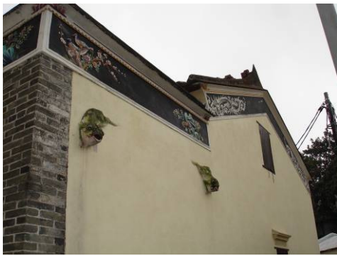
Plate 6b View of decorative wall details on No. 10 Wong Chuk Hang San Wai
