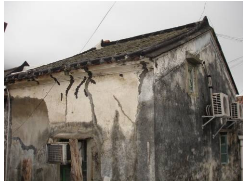
Plate 24b View of rear wall of House No. 17 Wong Chuk Hang San Wai
