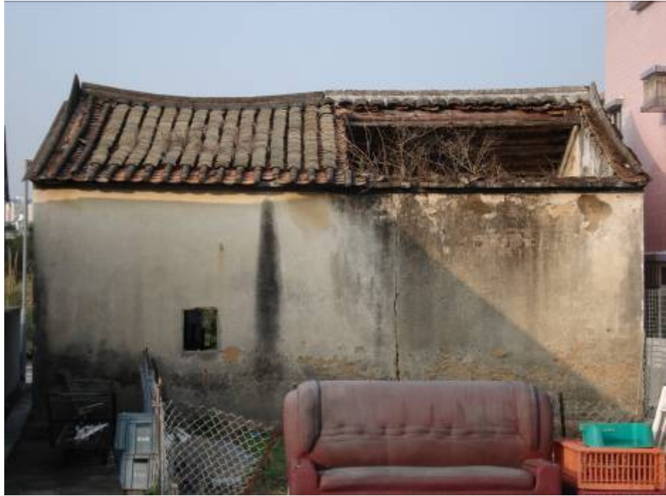
Back view (part of the roof has been collapsed)
