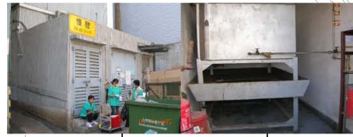
FUEL TANK ROOM AND EMERGENCY GENERATOR ROOM OF THE INTERNATIONAL MAIL CENTRE
