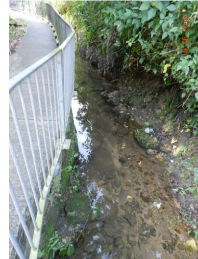
Plate 11. Watercourses present in the northeast and east of the Assessment Area are semi-natural to natural, usually with a retained natural bottom and sometimes partly concrete-lined (e.g. a watercourse in Tan Shan).
