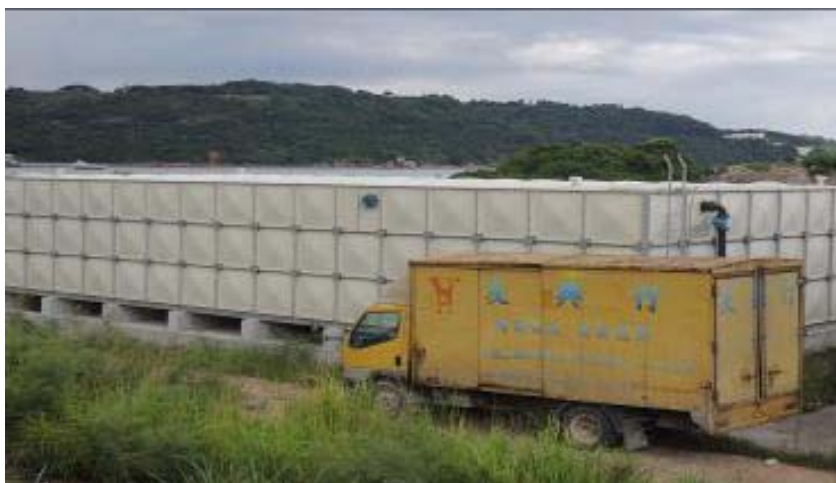
Fire Hydrant Tank adjacent to the Generator Room
