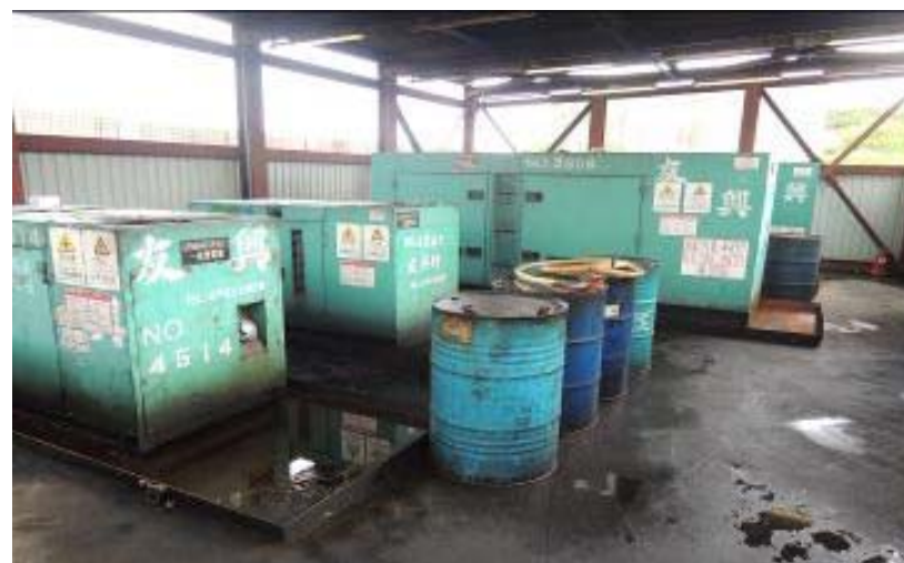
Generators inside the Generator Room.
