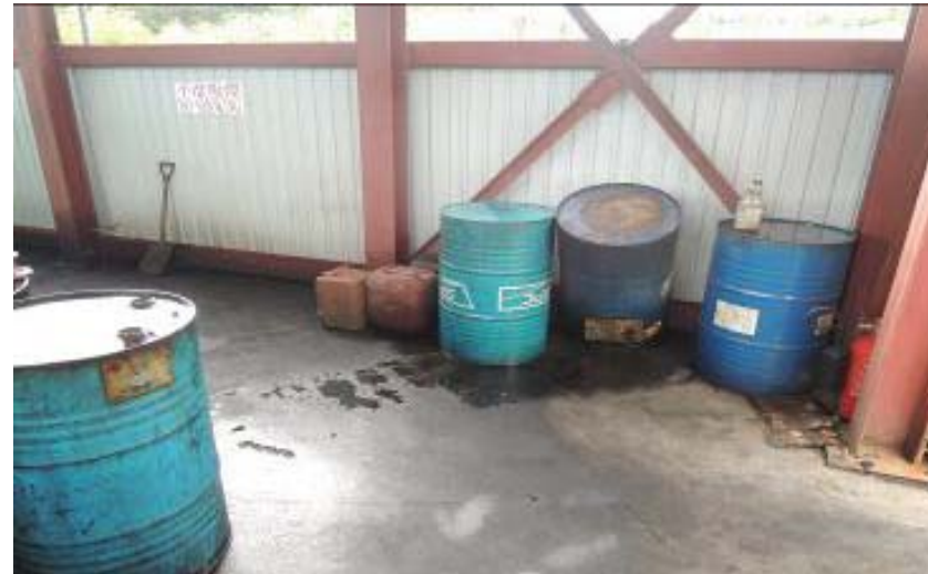
Diesel oil drums stored in the Generator Room without secondary containment
