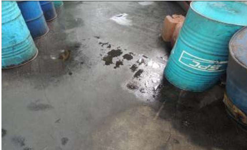
Oil stains observed on the paved ground of the Generator Room.
