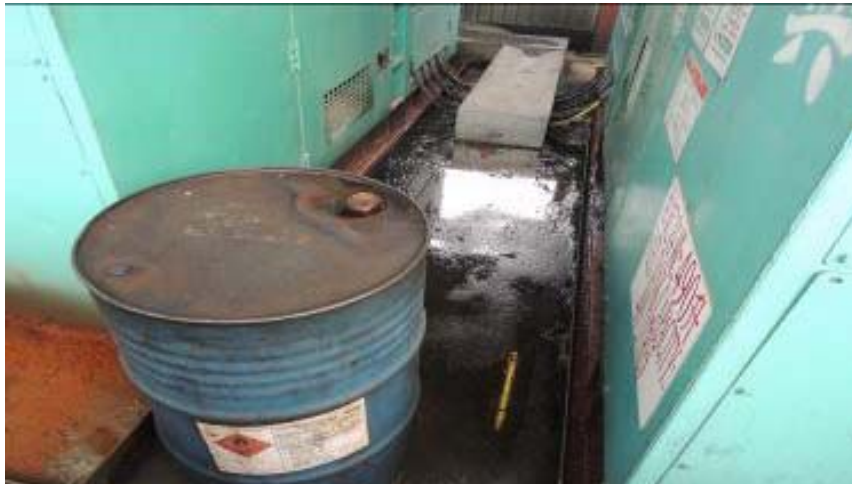
Oil spills next to the generators.
