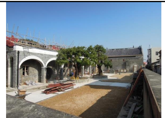
Yau Kung School main building of Tang Ancestral Hall, Ha Tsuen Shi (Declared Monument)
