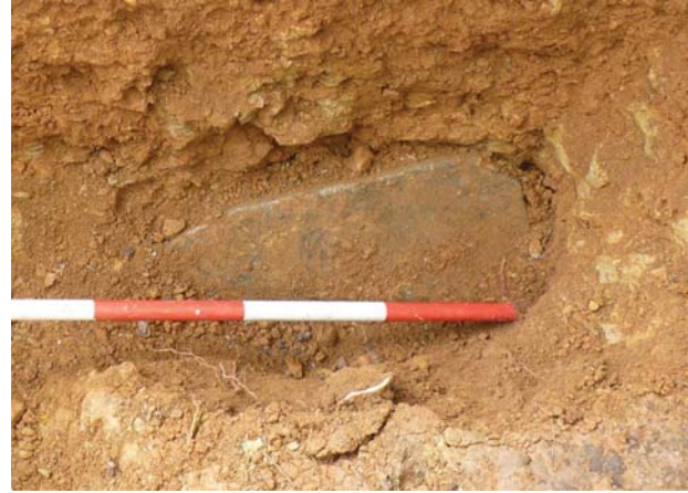
Plate B.17 Concrete cover and cable at bottom of hand excavated pit
