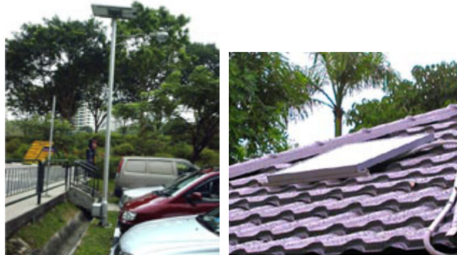
Examples of photovoltaics installations in Singapore 87
