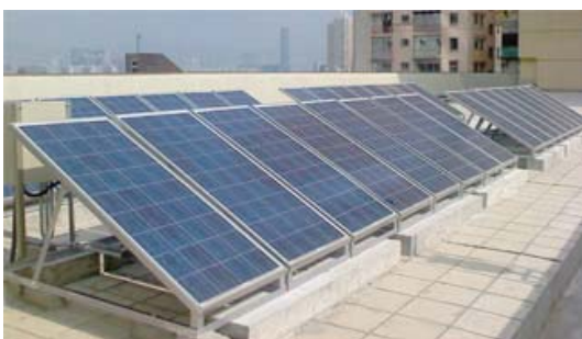
This set of solar panels, installed on the roof of a school, is an example of the minor works projects funded by the ECF.
