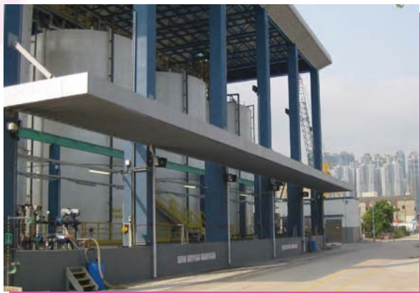
Disinfection facilities at Stonecutters Island STW
