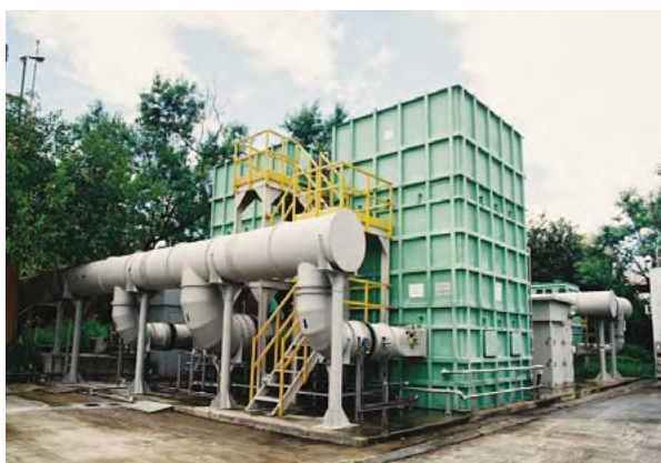
Deodourisation unit at Shatin STW
