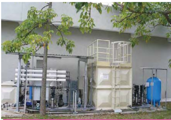
Reverse Osmosis Plant at Yuen Long STW
