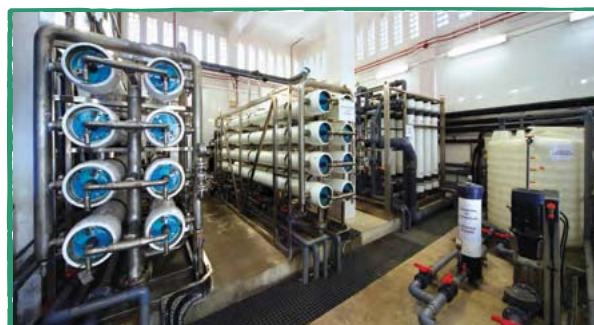
Effluent reuse treatment units next to the Water Reclamation Information Centre at Shatin STW
