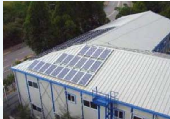
Photovoltaic power system at CRE's office
