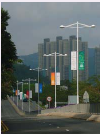
Special Carriageway Lighting
