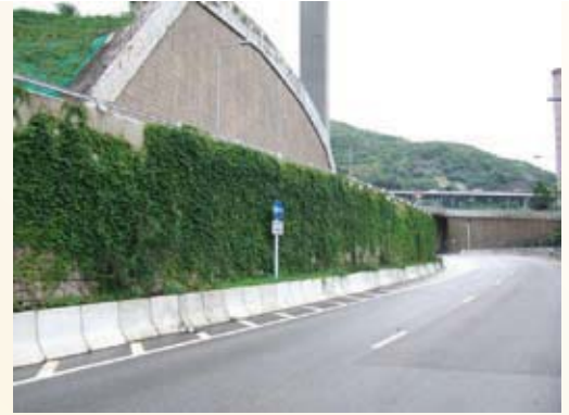
Greening on Retaining Wall at Castle Peak Road (Ting Kau)
