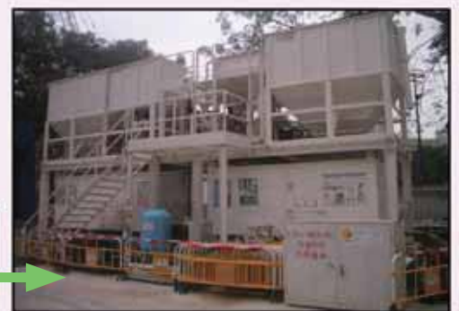
Waste water treatment system
